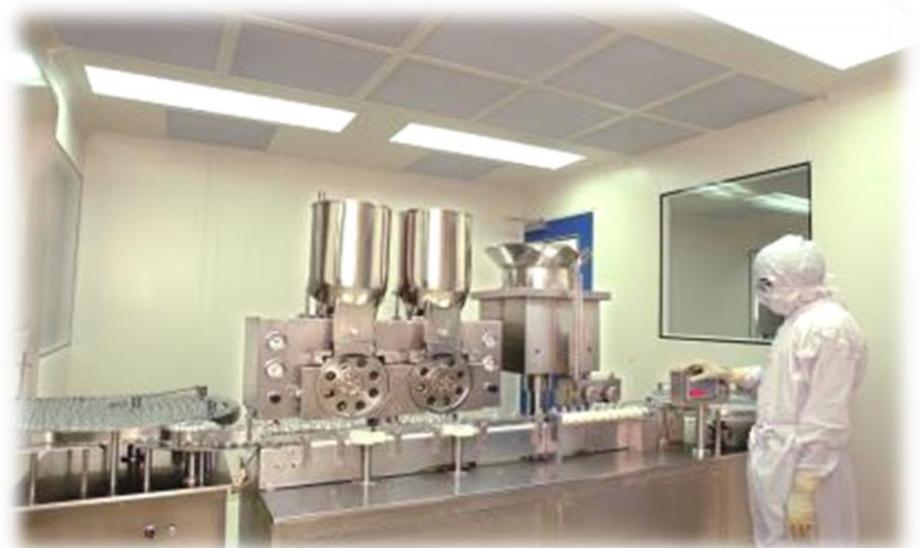
Production Area – Filling plant
